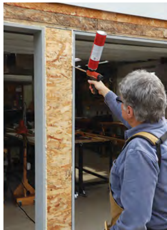
Foam the seams. Hartman applies foam sealant around the perimeter of the jambs. He'll add more to these spaces from inside.
