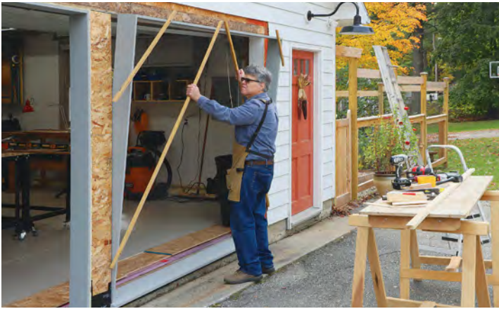
Square and set the jambs. After assembling the jambs in the shop, Hartman screwed on diagonal sticks to keep the jambs square and also to act as depth stops against the sheathing.
