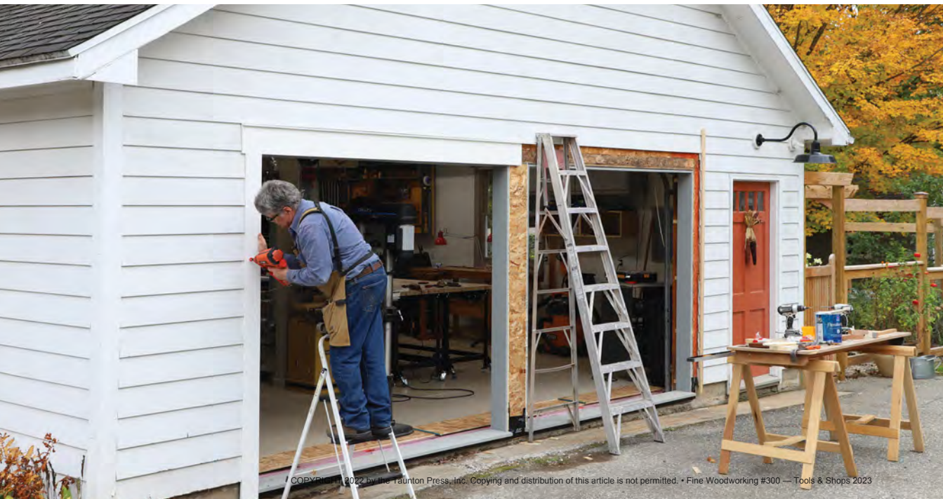
Casing the joint. Before hanging the doors, Hartman installs the casings around the opening. He used cellular PVC for its weather resistance.
